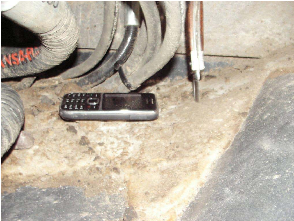
10. Inside and around battery
